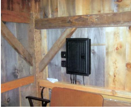
New Barn Electric Service Panel
