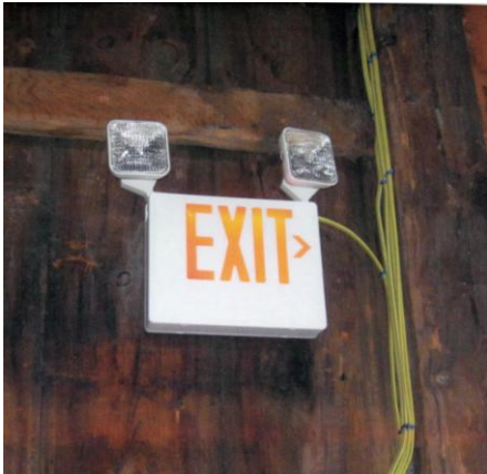
New Emergency Lighting
