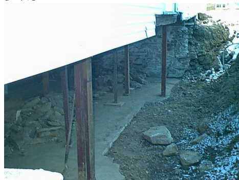
Barn construction site showing removed foundation wall and exposed rotted sill. (Photo by Bob Ducharme)
