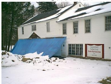
Stabilizing the front wall of the barn foundation (photo by Bob Ducharme)
